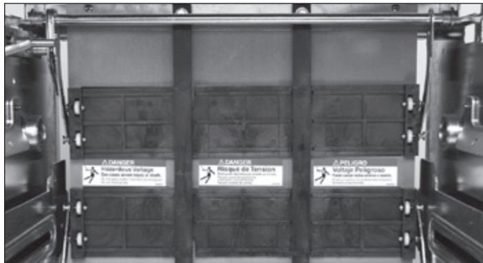
Figure 56. Safety Shutters in CLOSED Position
