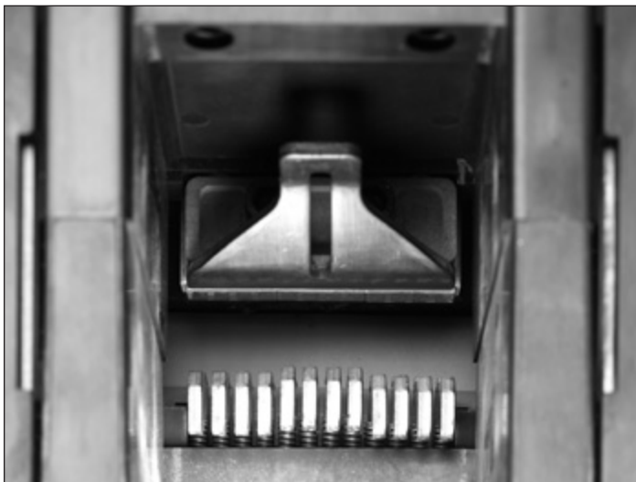
Figure 69. Primary Contacts with Circuit Breaker Open (Not Used for Contact Wear Inspection)
