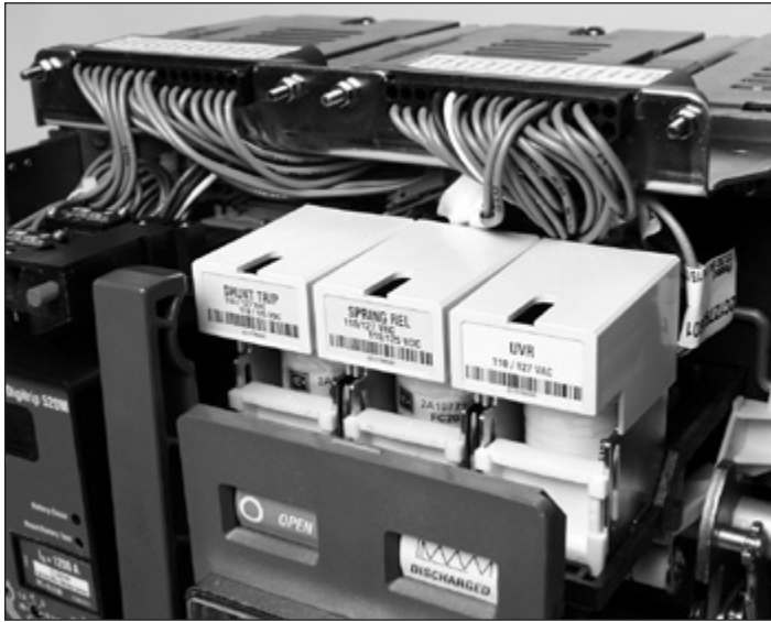
Figure 48. Shunt Trip, Spring Release, and Undervoltage Release Installed
